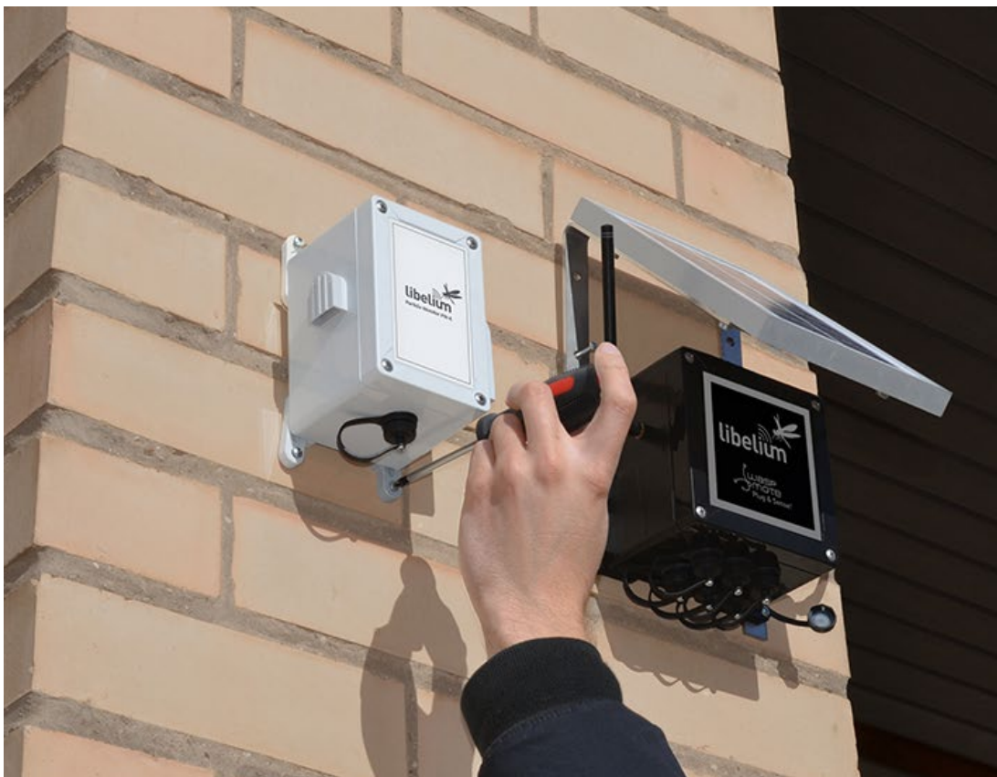
Figure: Fixing the Particle Matter – Dust Sensor Probe on a wall
